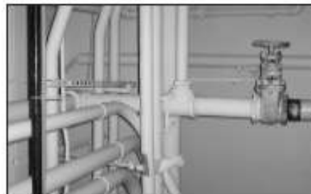
Piping and plumbing systems
